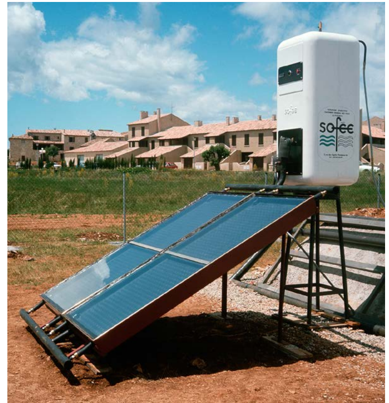
This solar water heater is one of many used to heat water for the town of Méjannes-le-Clap, France.
